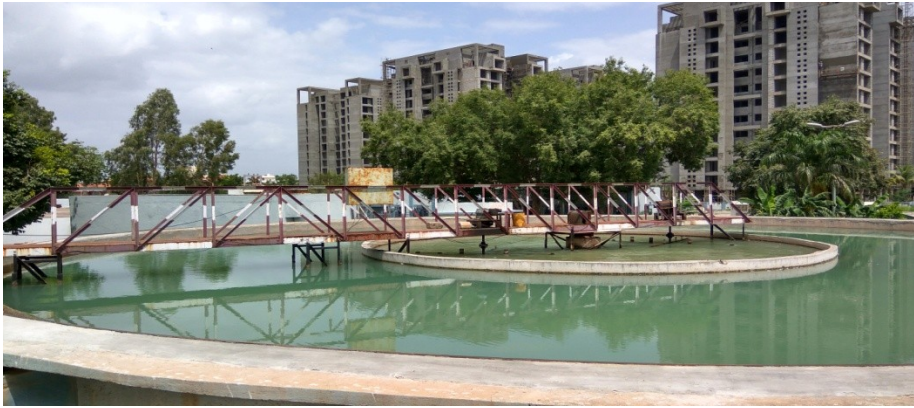
“Clariflocculator view of purified water”
